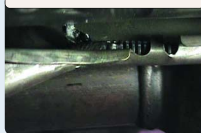
Location of damage
